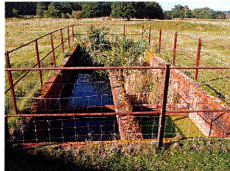
Right - F.F.D 1 – Brick mixing tank used for the collection of effluent for treatment prior to discharge to soakaways. © by Graham Smith 2007
