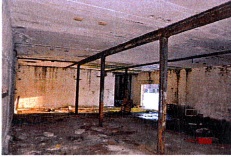
Left: A View inside from inside one of the charging buildings showing the stations and steel beams, also visible in the roof adjacent to the closest beam are three holes where the vesicant pipes fed through from the tank above. © by Graham Smith 2010
