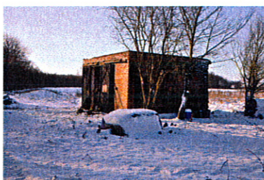
Left – F.F.D 2 the sole remaining building on the site at time of writing this being the emergency de-contamination building . © by Graham Smith 2010
